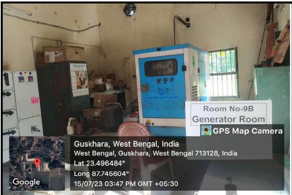
Figure-82: Generator Room
